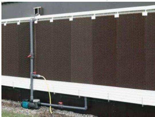
RainMaker pad-cooling system
